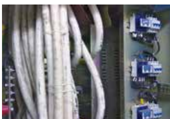
▲ Energy meter in a harsh industrial environment
