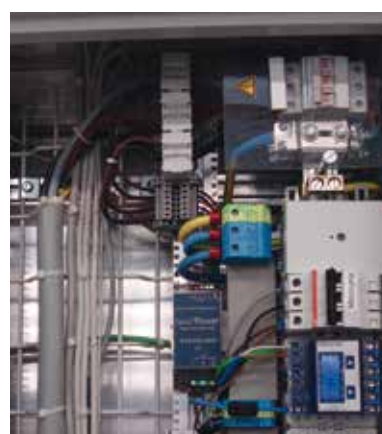
▲ Built-in current transformer in cable duct
